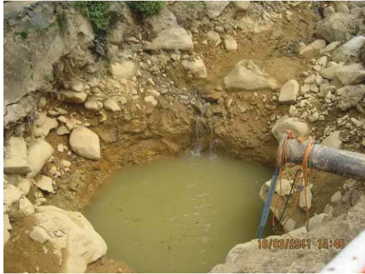
Fig.2.1 – Muddy water arisen from excavation at ch.200
