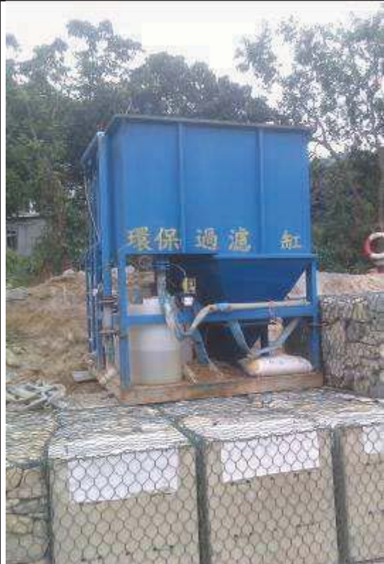
Fig.3.2 – Site water from construction activities at ch.400 was diverted to sedimentation tank (photo taken by Contractor)
