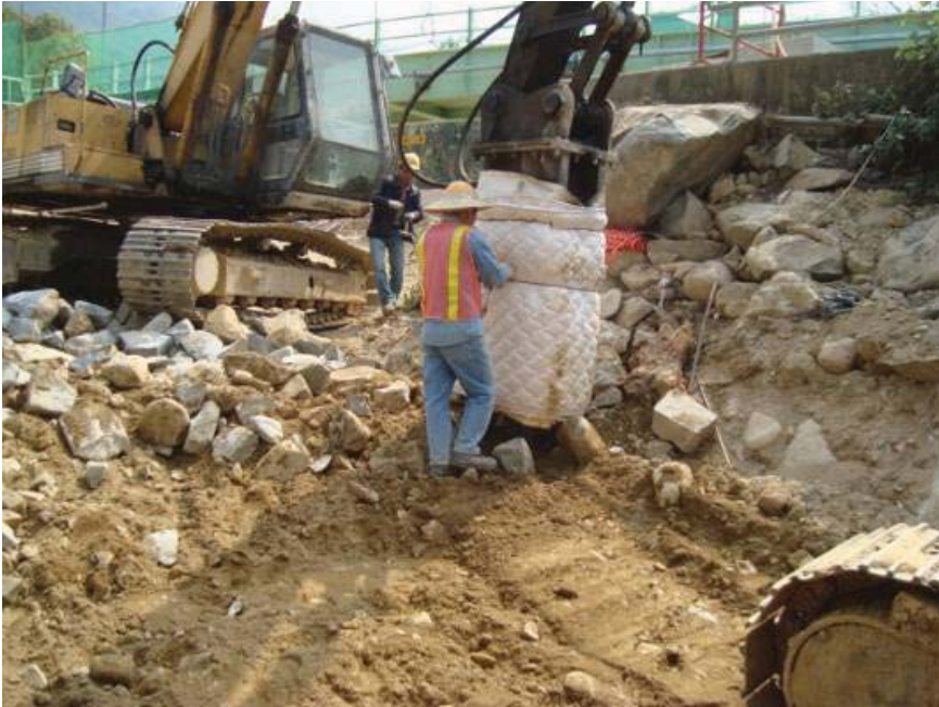
Fig.1 – Breaker Tips of Hydraulic Breaker was warped up with noise insulation material
