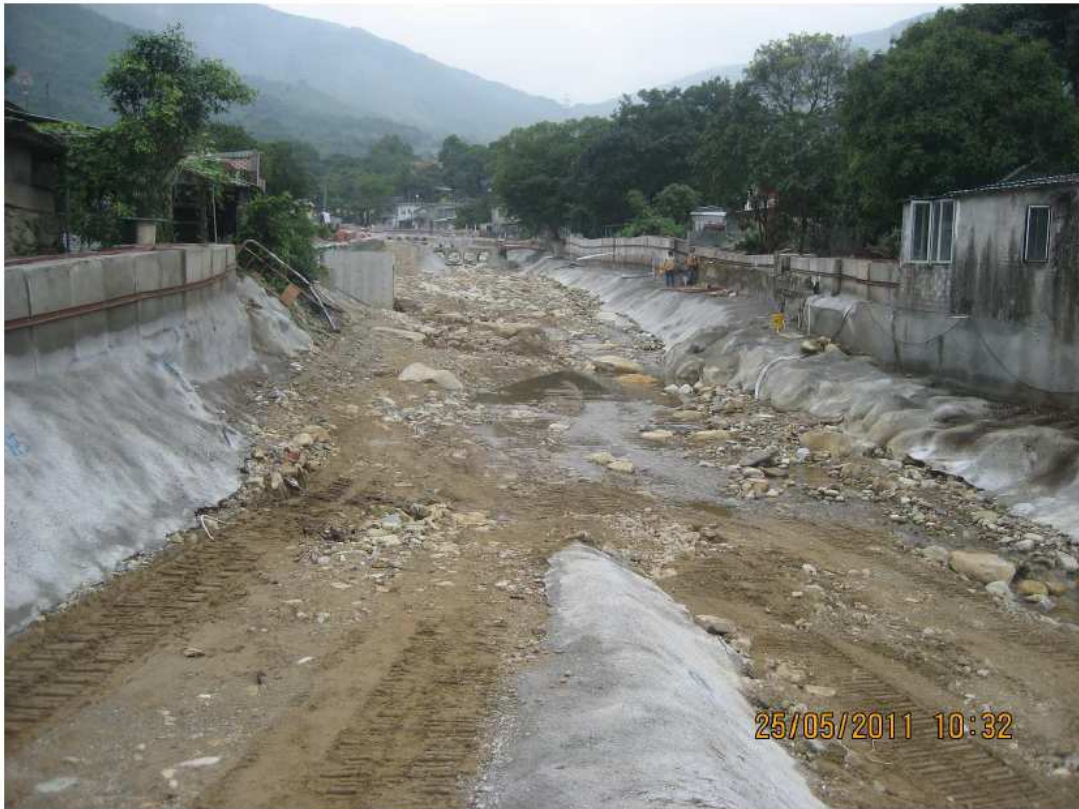
Fig.5.1 – During site investigation, no river work was being carried out between ch.400 and 500 of UTPR
