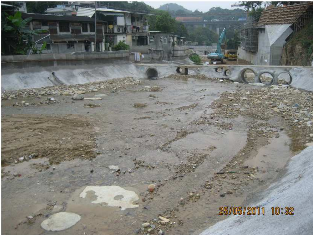
Fig.5.2 – During site investigation, no river work was being carried out between ch.500 and 600 of UTPR
