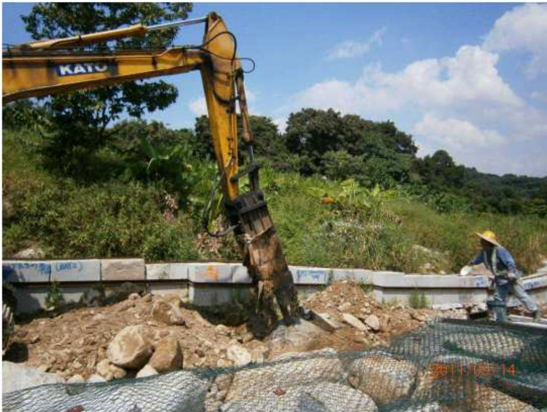
Fig 7.1 – During site investigation, water spraying was provided and the breaker Tips of Hydraulic Breaker was warped up with noise insulation material
