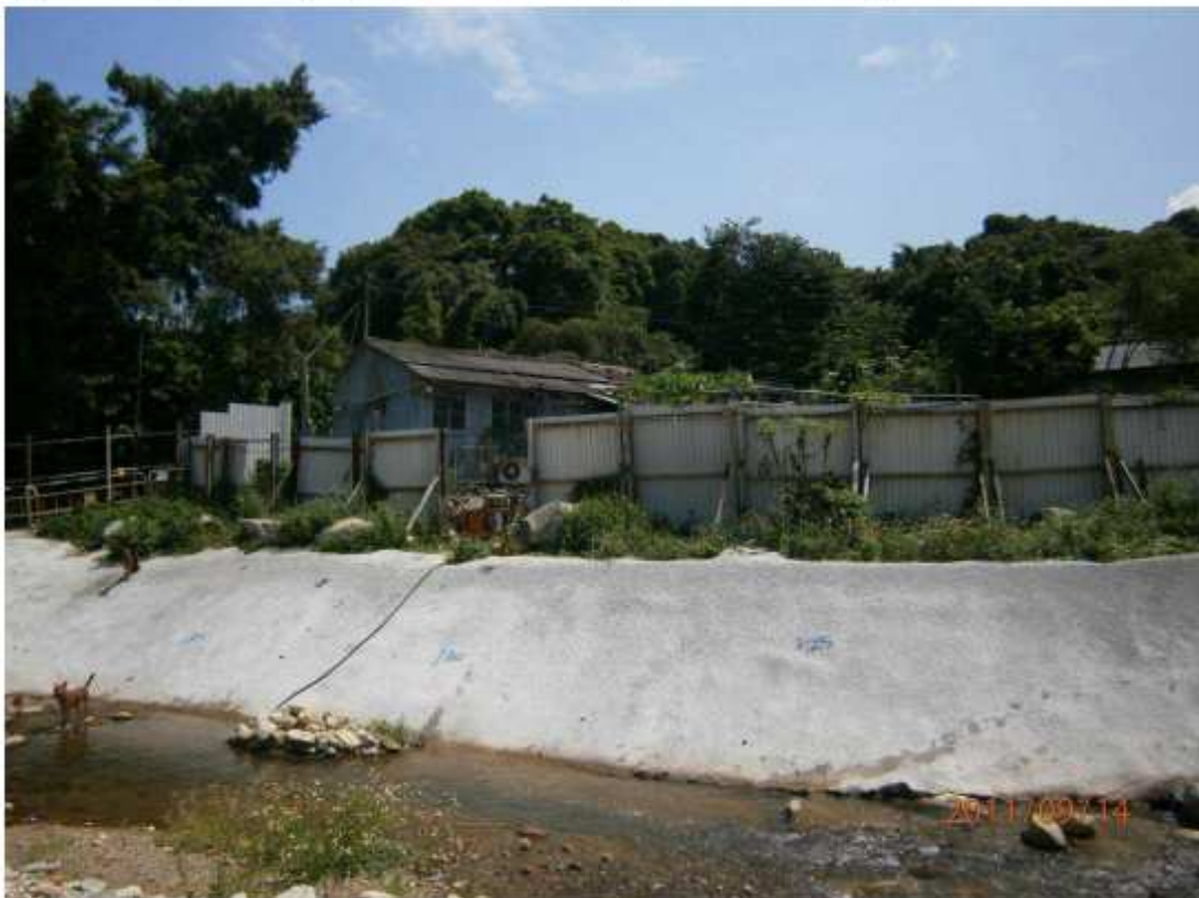
Fig 7.2 – During site investigation, noise barriers were set up near Sha Po Tsai Village
