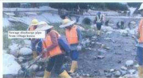
Photo 5: Sewage discharge pipe
