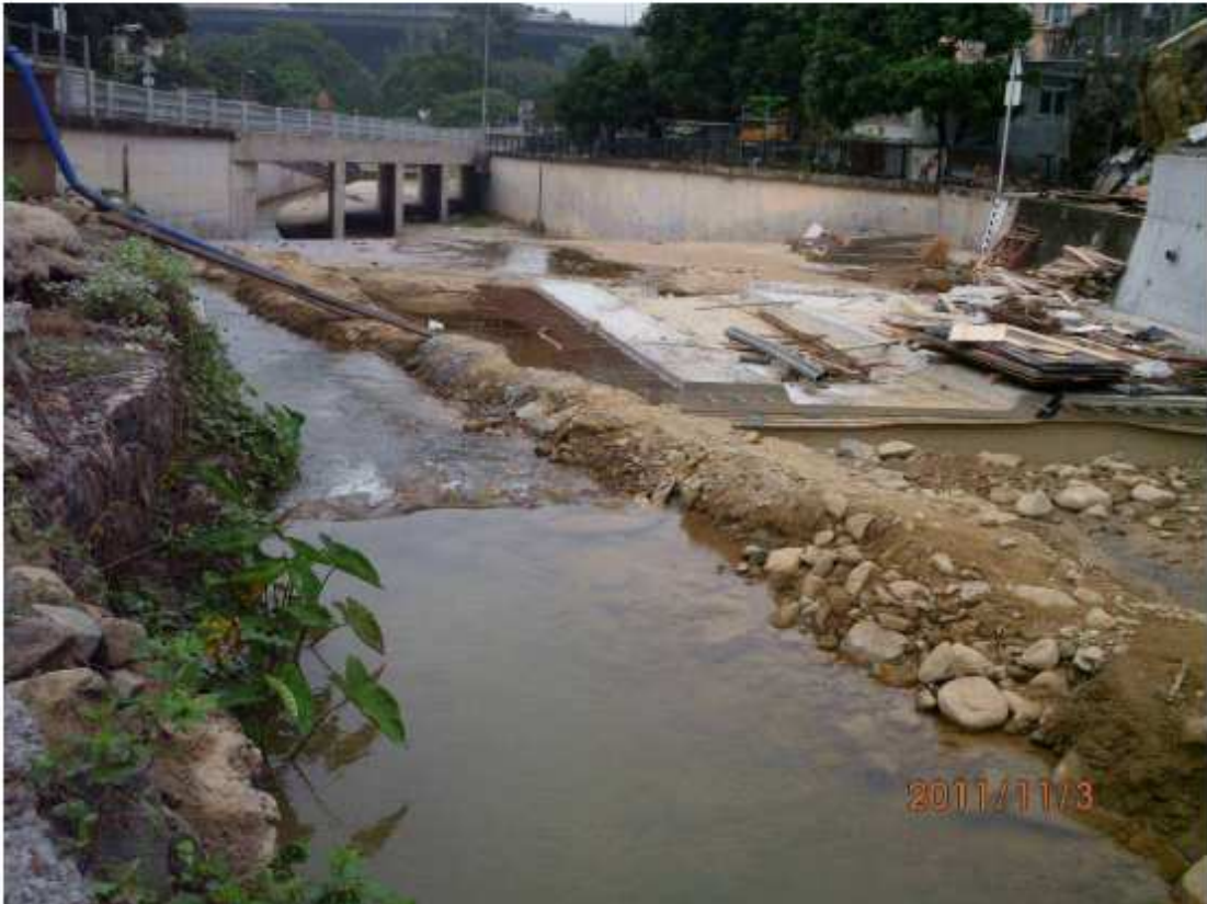
Fig.6.2 – The river quality was acceptable with no muddy water observed (photo provided by Contractor).
