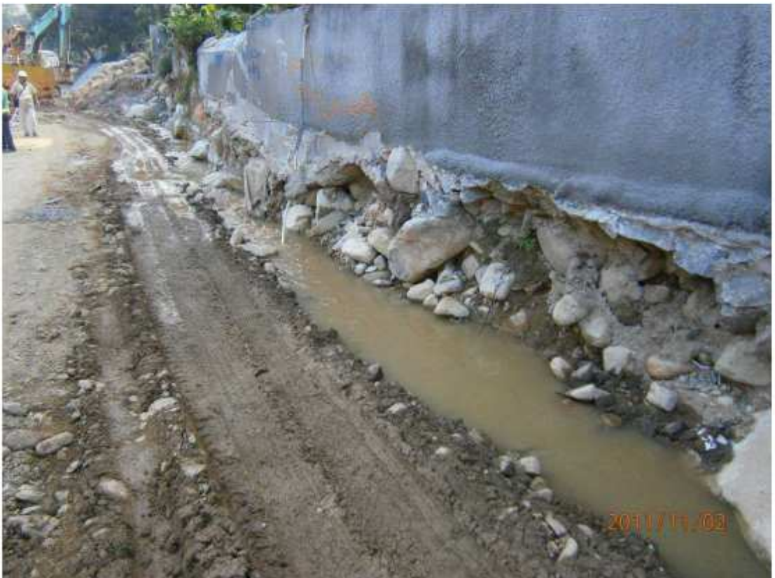
Fig.5.2 – Muddy surface runoff caused by seeping of underground water and domestic waste water.
