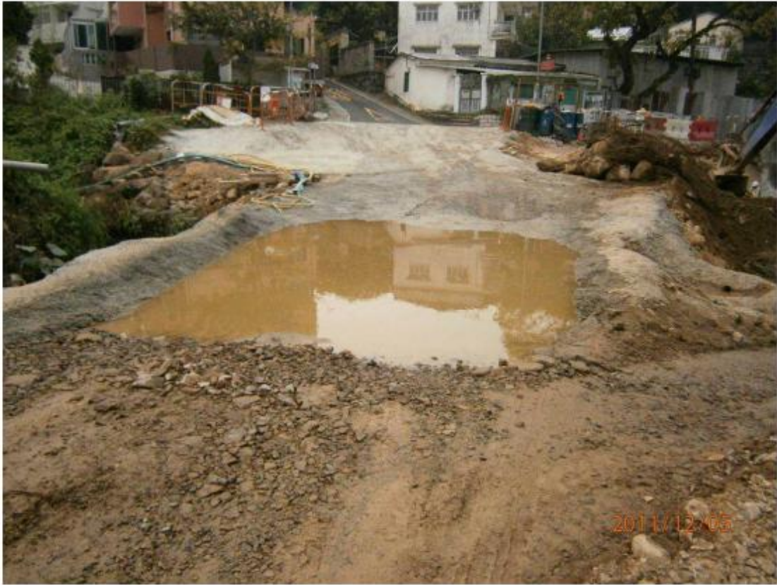
Fig.5.2 –Condition of Wheel Washing Bay at site entrance located at ch.600 was muddy.
