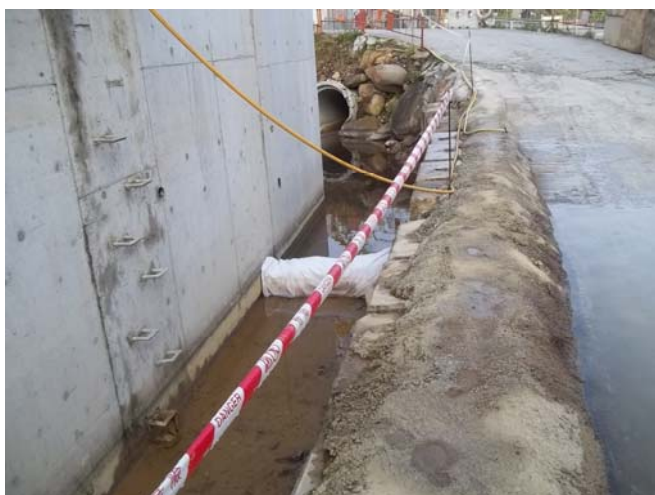
Photo 4: At spot 2 near CH550, earth bund has been constructed in order increase the sedimentation time of river water. No muddy water was observed at Spot 2 on 16 January.
