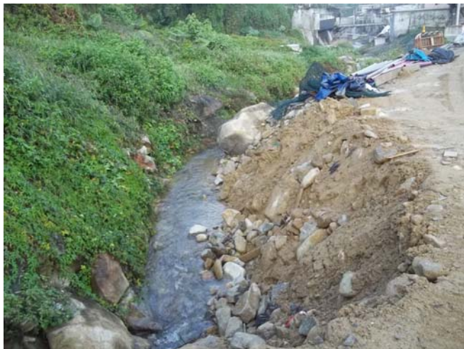
Photo 3: No muddy water was observed at Spot 1 on 16 January.
