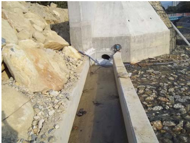
Photo 2: Sand bags were placed near inlet of dry weather channel at area CH100 to prevent muddy water flowing into the downstream of UTPR.
