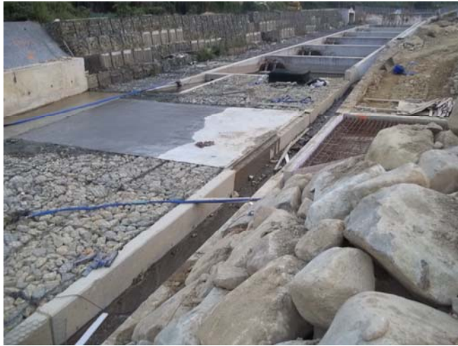
Photo 1: The loose soil at the exposed construction work area near area CH100 was removed and that exposed area has been became a concrete surface. No muddy water was observed at Spot 1 on 16 January.
