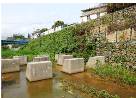
Photo 4: Vegetation growing on gabion (Middle section)
