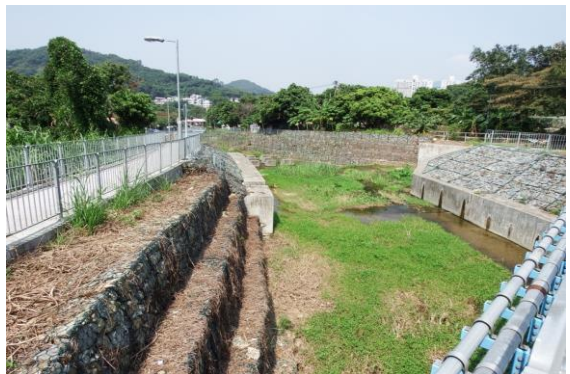
Photo 4: Vegetation sparsely growing on gabion and river bed
