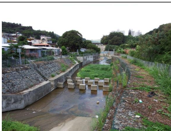
Photo 4: Vegetation sparsely growing on gabion and river bed
