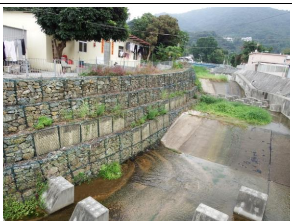
Photo 4: Vegetation sparsely growing on gabion and river bed
