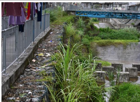
Photo 4: Vegetation sparsely growing on gabion
