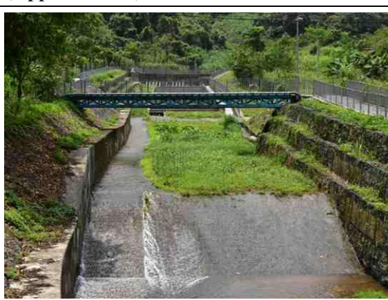
Photo 4: Vegetation sparsely growing on gabion
