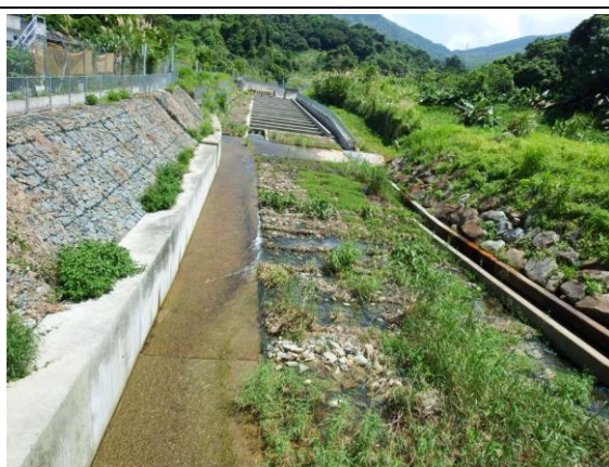
Photo 4: Vegetation sparsely growing on gabion
