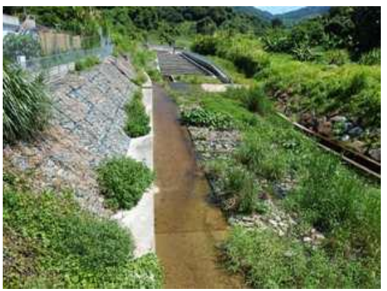
Photo 4: Vegetation sparsely growing on gabion (Middle section)
