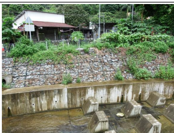
Photo 4: Vegetation sparsely growing on gabion (Middle section)
