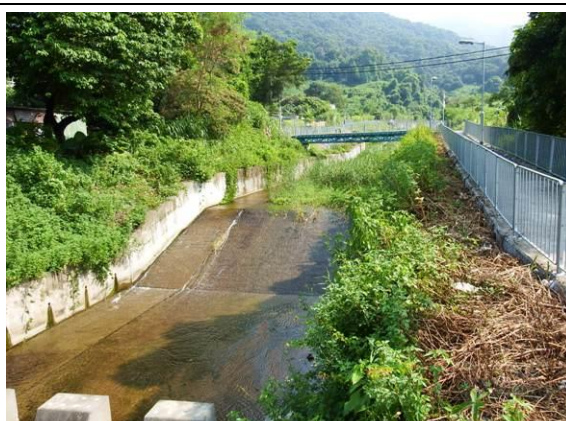
Photo 4: Vegetation sparsely growing on gabion (Middle section)
