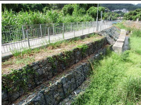
Photo 4: Vegetation sparsely growing on gabion (Middle section)
