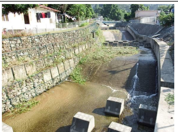
Photo 4: Vegetation sparsely growing on gabion (Middle section)
