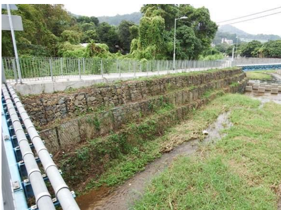
Photo 4: Vegetation sparsely growing on gabion (Middle section)
