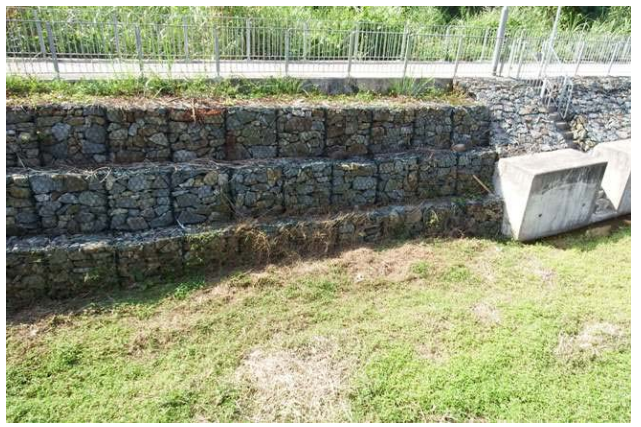
Photo 4: Vegetation sparsely growing on gabion (Middle section)
