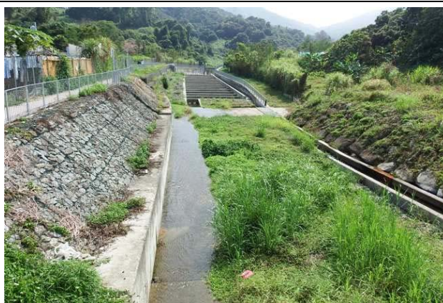
Photo 4: Vegetation sparsely growing on gabion (Middle section)
