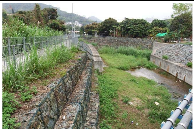
Photo 4: Vegetation sparsely growing on gabion (Middle section)
