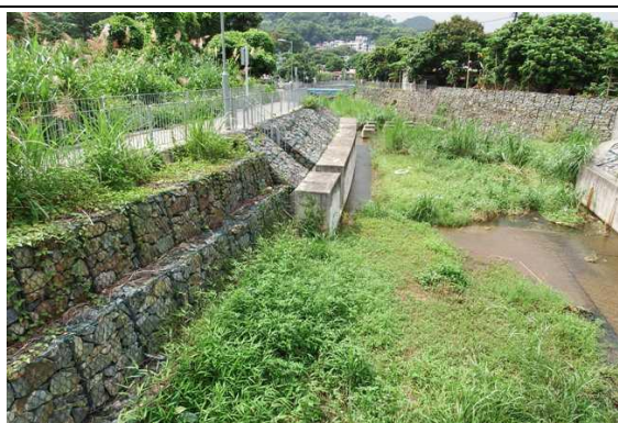
Photo 4: Vegetation sparsely growing on gabion (Middle section)
