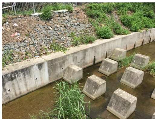
Photo 4: Vegetation sparsely growing on gabion (Middle section)
