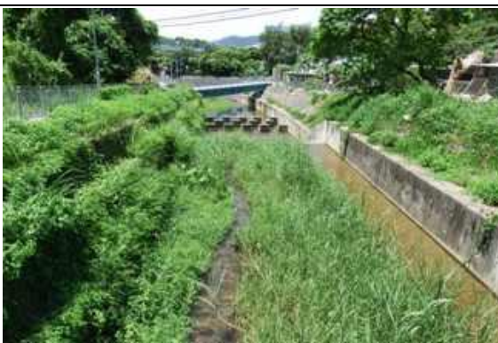
Photo 4: Vegetation sparsely growing on gabion (Middle section)
