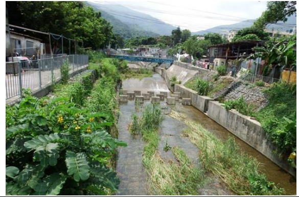
Photo 4: Vegetation sparsely growing on gabion (Middle section)
