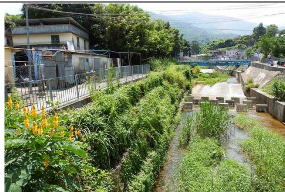
Photo 4: Vegetation sparsely growing on gabion (Middle section)
