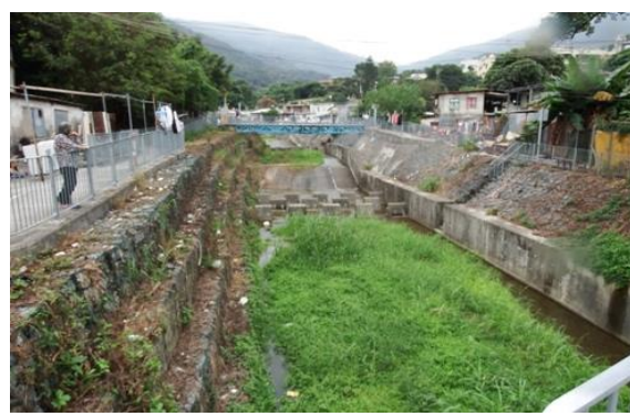
Photo 4: Vegetation sparsely growing on gabion (Middle section)
