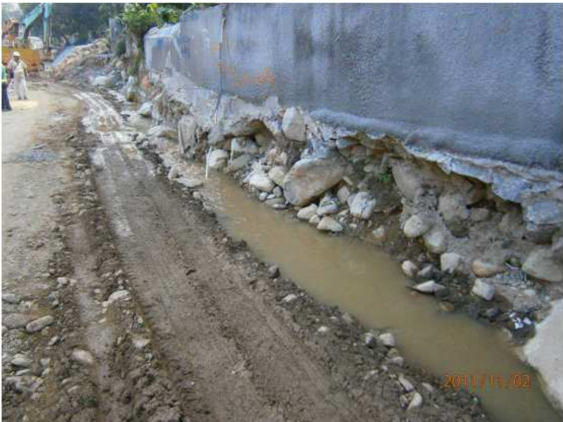
Fig.5.2 – Muddy surface runoff caused by seeping of underground water and domestic waste water.
