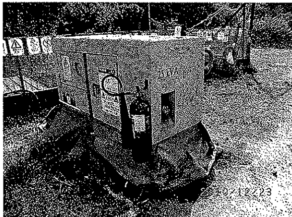
Photo 7 Water Filling Station No. 2 Oil was seeped from the drip tray.
