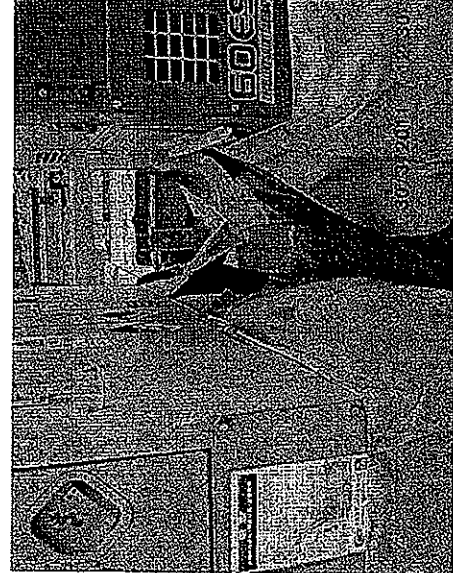
Photo 110330_011 (Generator at weighbridge near Pier No.1)
