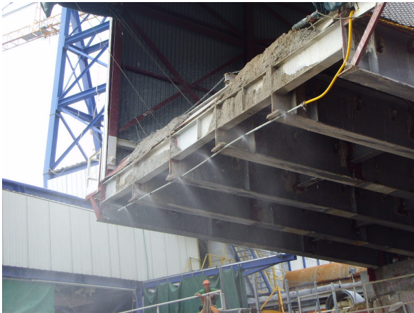
Photo 9: Sprinkler system installed at the ramp jetty
