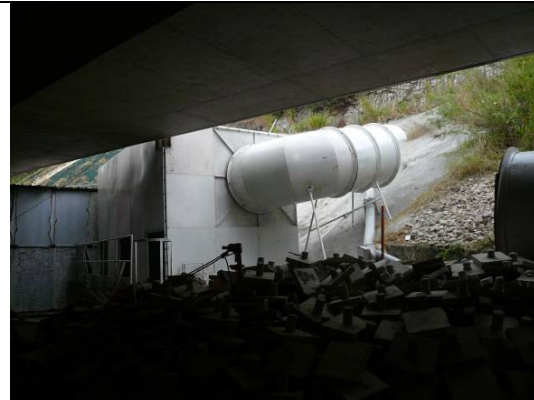
Fume scrubber in the Western Portal
