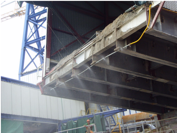
Photo 9: Sprinkler system installed at the ramp jetty
