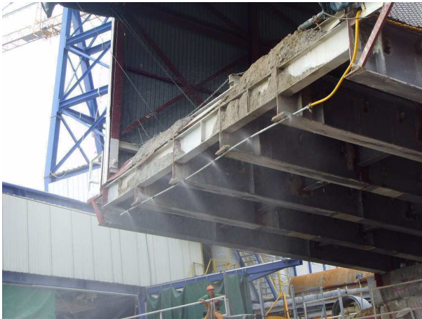
Photo 9: Sprinkler system installed at the ramp jetty
