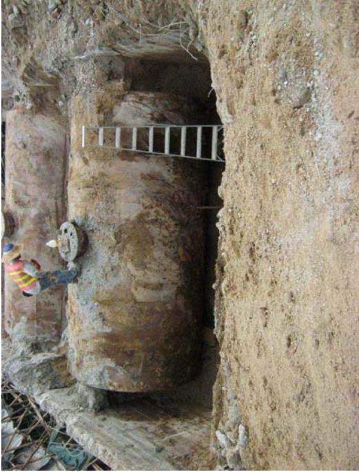
Photo 1: A view of Kerosene Tanks inside the Concrete Box Containment
