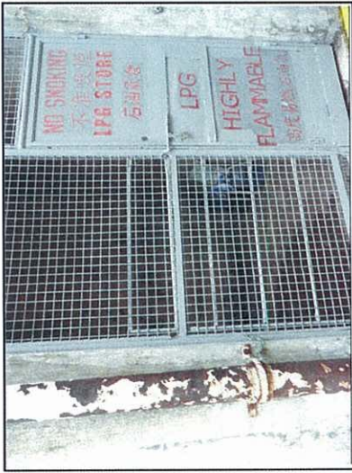
Photo 13: A DG store was found near the entrance of Ground Floor. The store was concrete paved with no crack. No LPG container or stain was found within the store.
