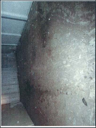
Photo 2: The floor slab of the Roof Floor was concrete paved. No visual evidence of spillage/staining was observed.
