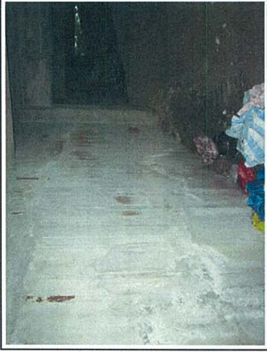
Photo 9: The wall of concrete box containment on Underground Tank Level was exposed to air. The concrete box is used to hold the three tanks inside.
