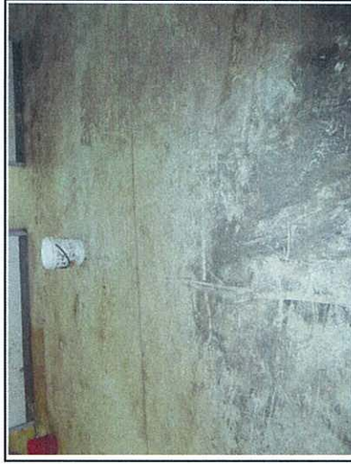
Photo 5: The floor slab of the Lower Ground Floor was concrete paved. No visual evidence of spillage/staining was observed.
