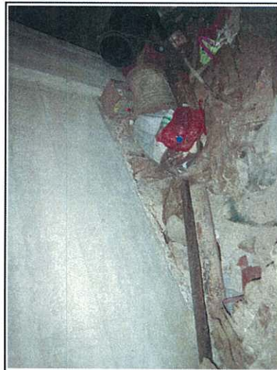
Photo 10: The concrete box containment was placed on a layer of filled rocks.
