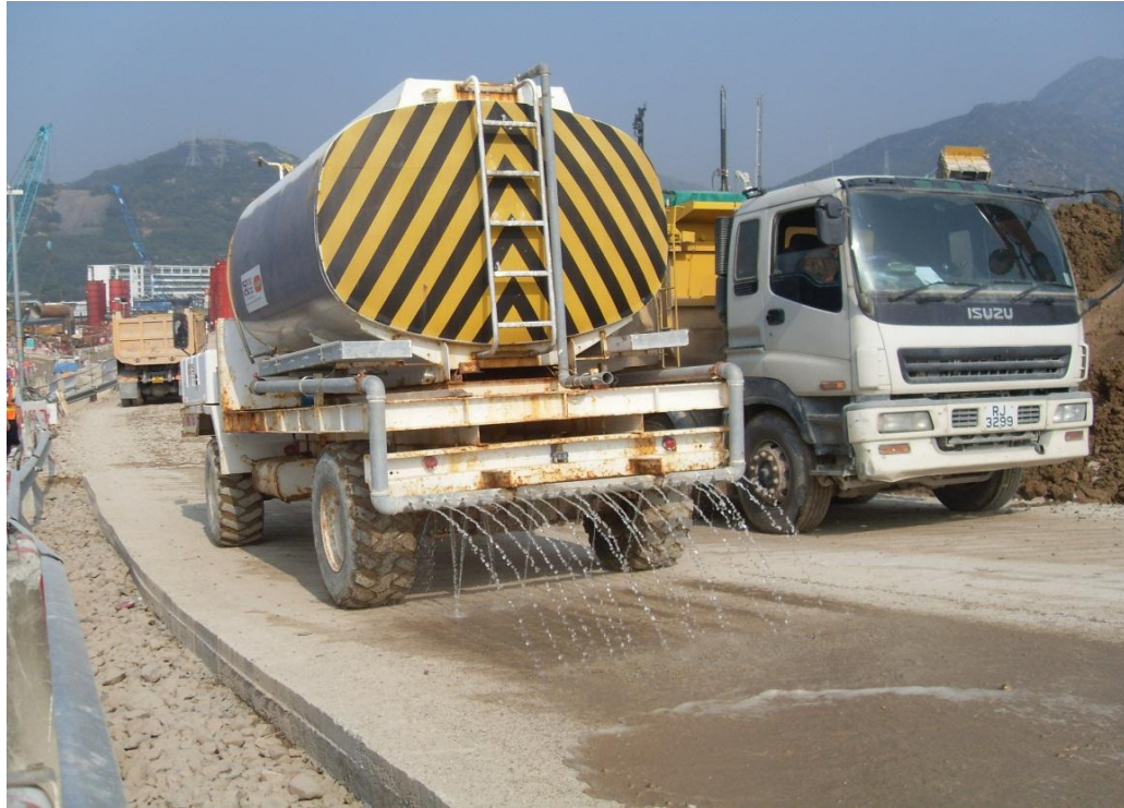
Water truck was observed in used during site investigation. (Reclamation Works Area)
