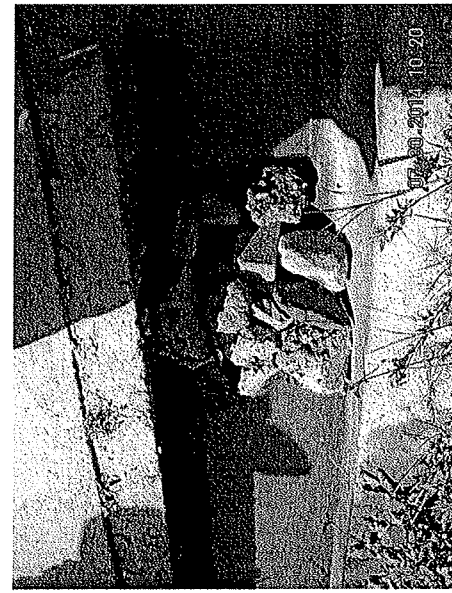
Photo 140730_005 (Catchpit CP5 and CP8)
