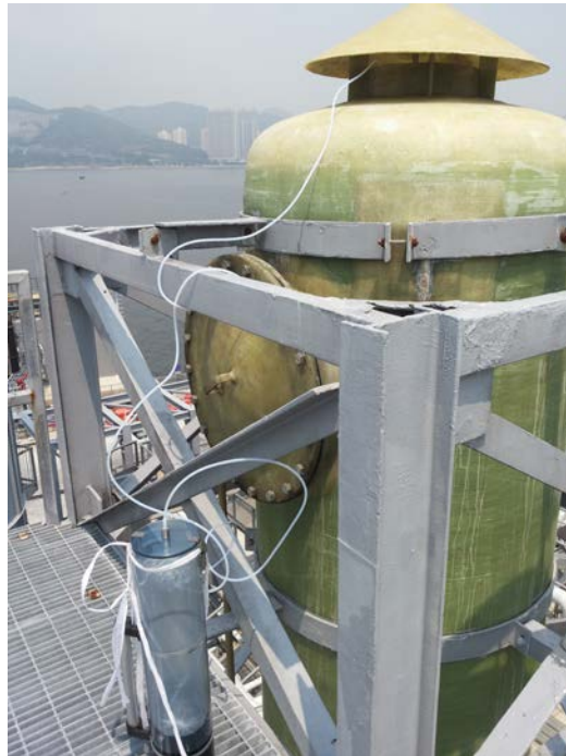
Final air scrubber
