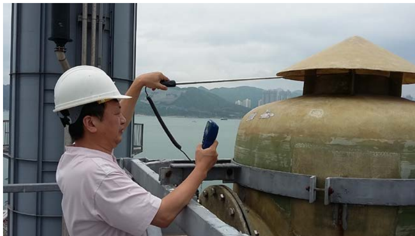
Final air scrubber
