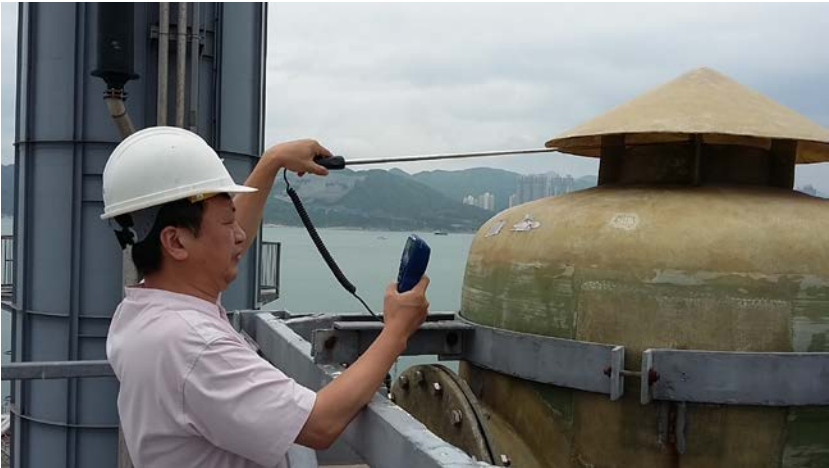
Final air scrubber
