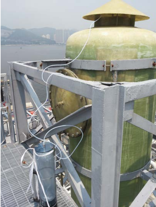
Final air scrubber
