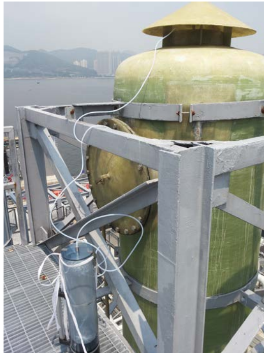
Final air scrubber
