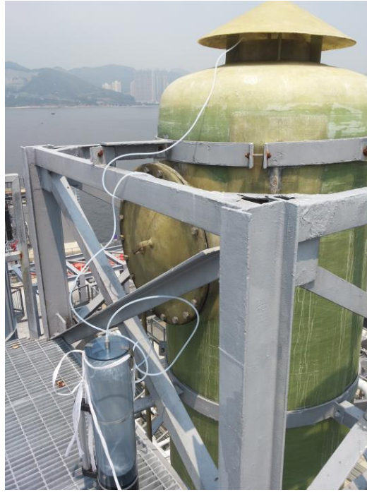
Final air scrubber
