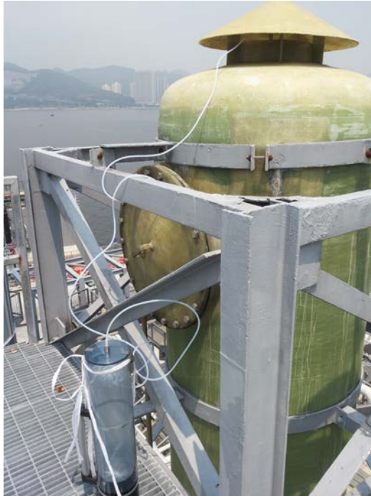
Final air scrubber
