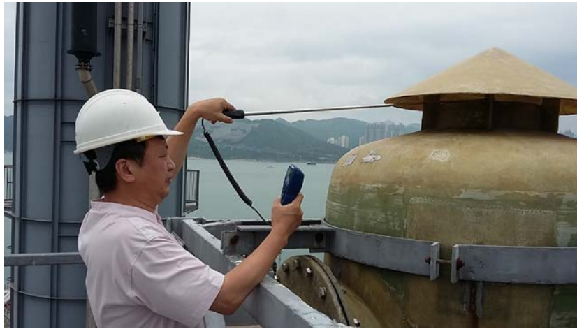
Final air scrubber
