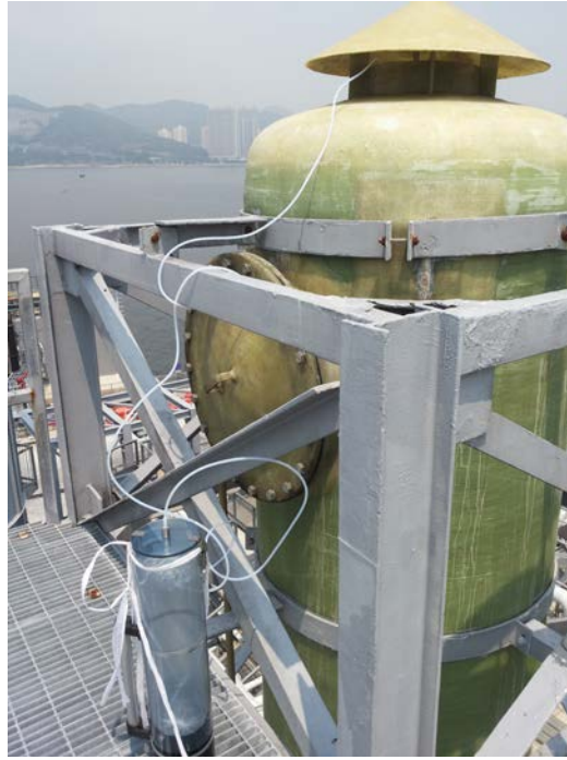
Final air scrubber
