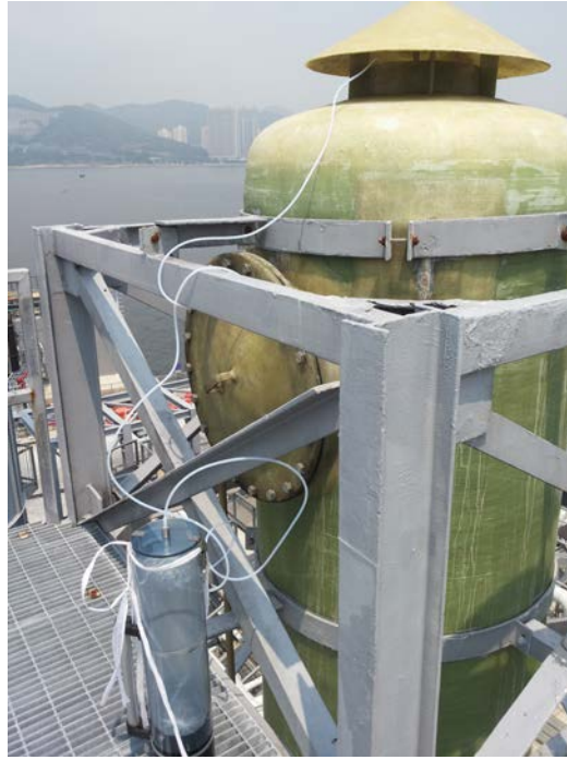
Final air scrubber
