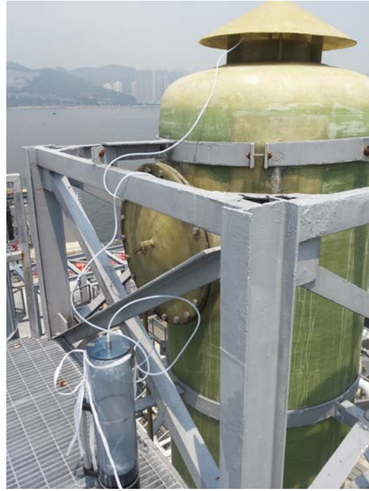
Final air scrubber
