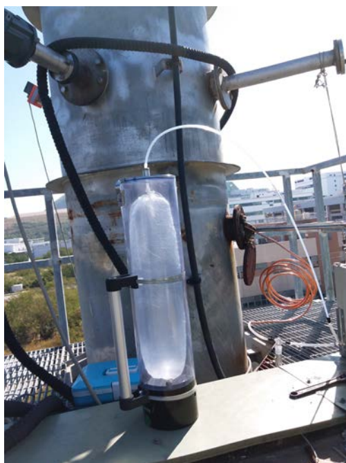
Boiler stack (EP2)
