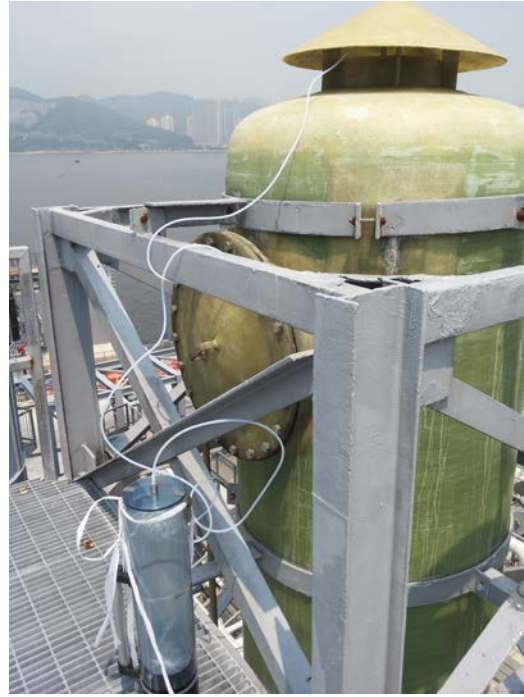
Final air scrubber
