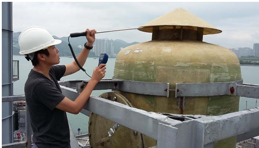
Final air scrubber
