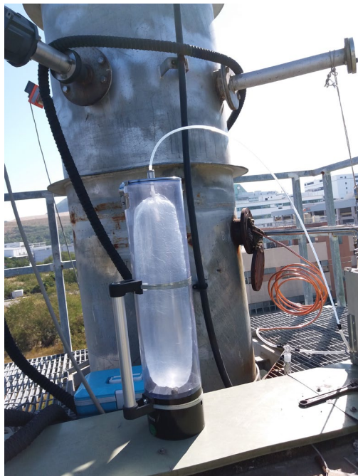
Boiler stack (EP2)
