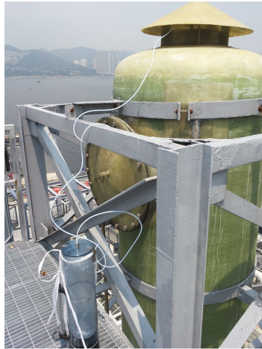
Final air scrubber
