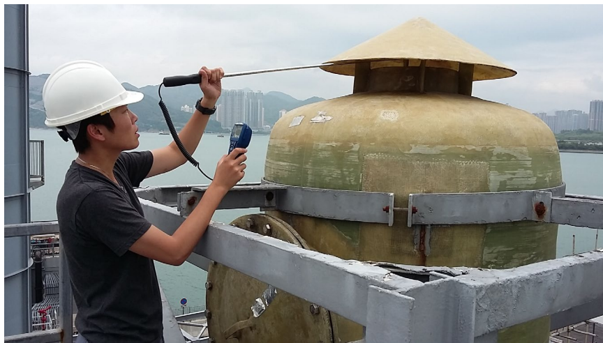
Final air scrubber
